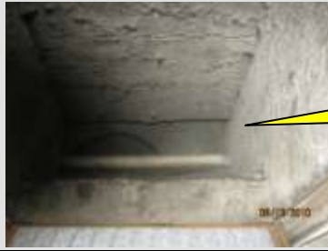
Dust buildup inside return air
